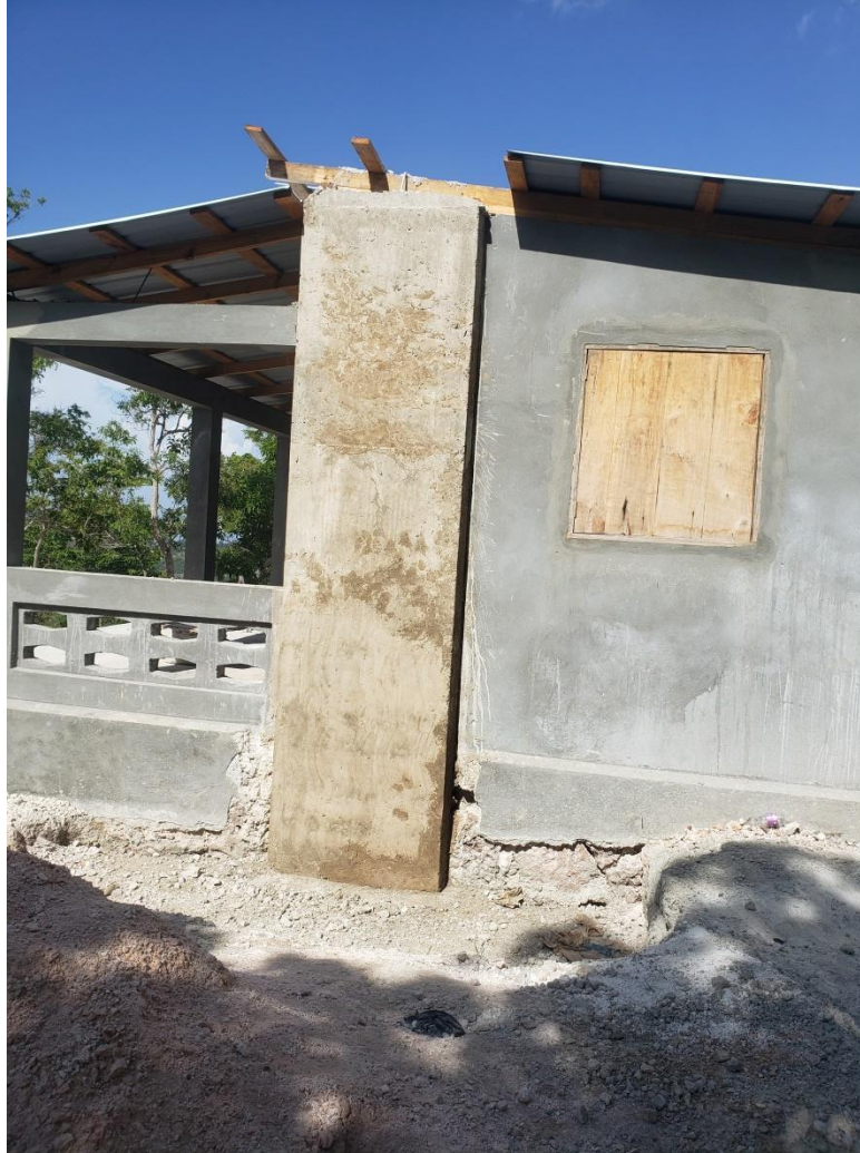
Figure 8. Concrete shear wall observed condition after removal formwork. Buidling 2
