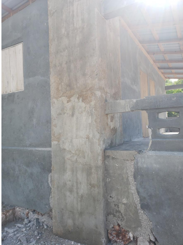
Figure 7. Concrete shear wall observed condition after removal formwork- Buidling I.
