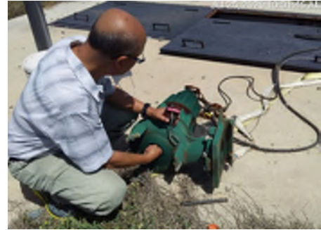
AECOM'S MEP ENGINEER INSPECTED DAMAGE TO LIFT STATION PUMPS AND DEVELOPED SOLUTIONS IN COLLABORATION WITH HOME OFFICE SPECIALISTS
