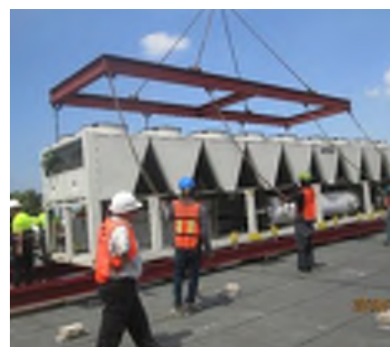
AFTER IDENTIFYING STRUCTURAL ISSUES WITH THE ROOFTOP CHILLER INSTALLATION, AECOM SUPPORTED USAID IN IDENTIFYING SOLUTIONS TO PROGRESS THE PROJECT
