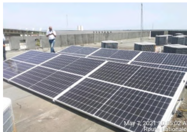
AECOM MEP ENGINEERS PROVIDED INSPECTION OF THE LIMONADE UNIVERSITY SOLAR PANELS SYSTEM PROJECT PRIOR TO USAID'S ISSUANCE OF A CERTIFICATE OF COMPLETION
