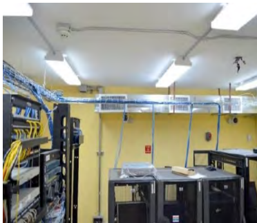
After the NOC's renovation, servers and cords are clearly organized and easier to access.
