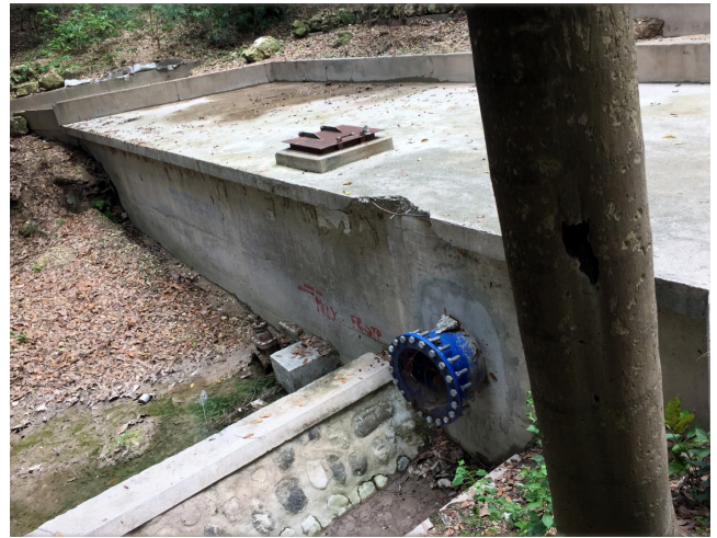
Photo 10. Outside view, overflow portal to surface drainage.
