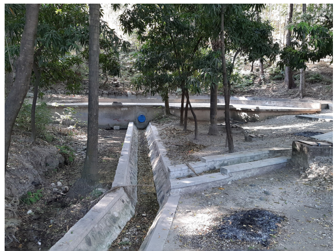
Photo 18. Overflow and drainage canals leading from catchment.
