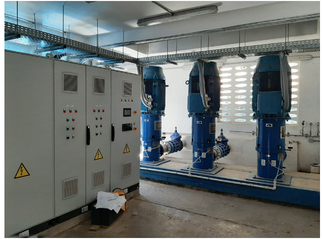
Photo 4. Source Mariani pumping station.
