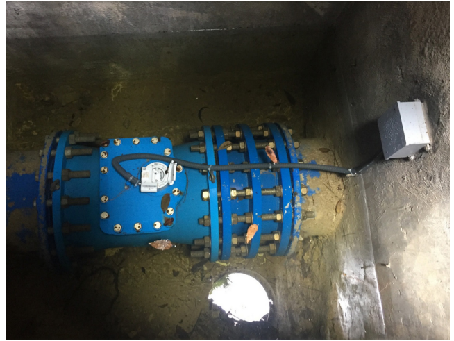
Photo 14. Totalizing flow meter measuring spring flow to pumping station.
