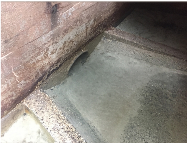
Photo 11. Historical washout portal.
