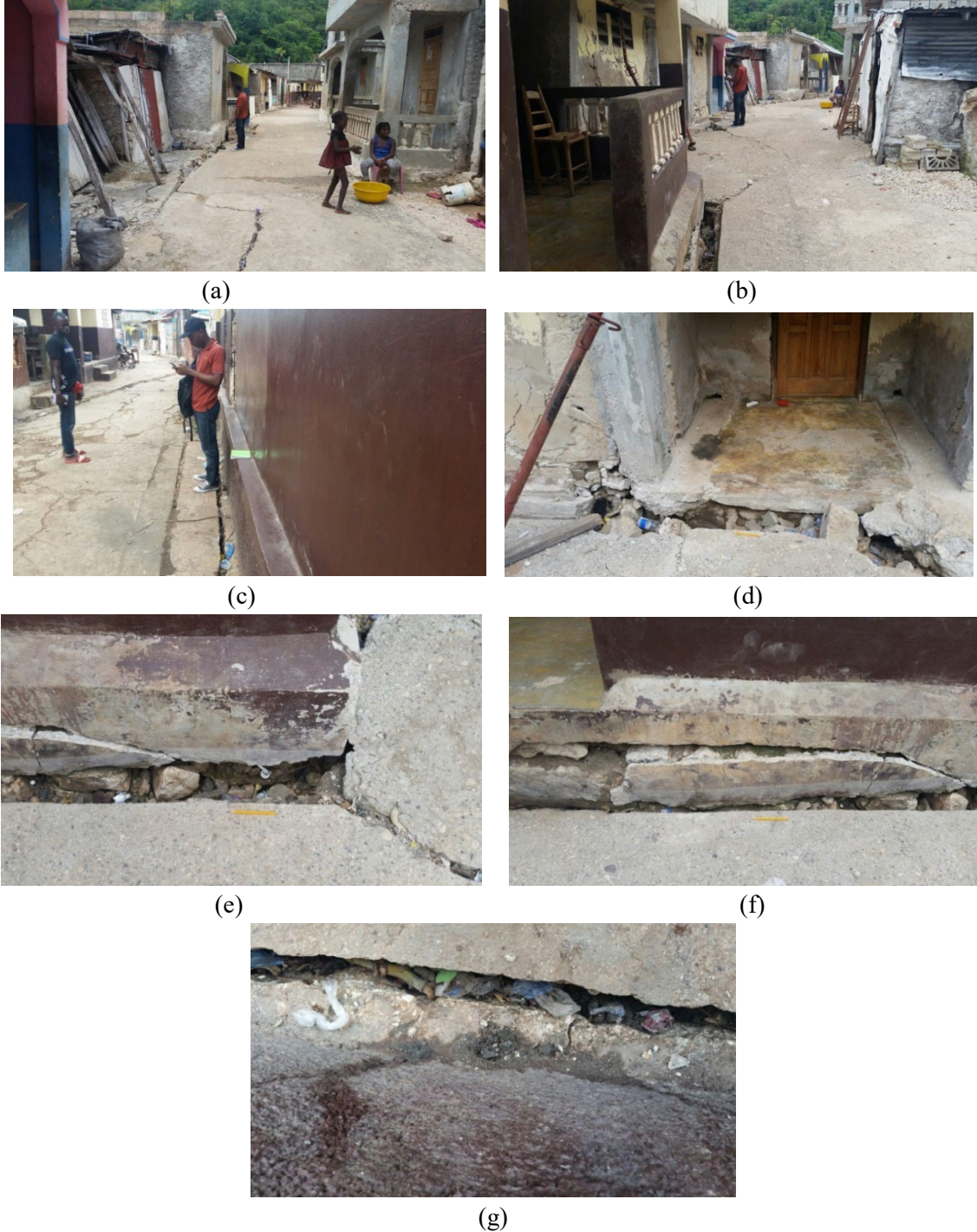
Figure 7.82. Reported observations of liquefaction during the August 14 th Nippes Earthquake (Lat: 18.5435502, Lon: -73.7921043).
