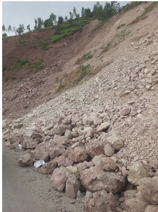
Figure 7.30. Rockfall along RN7 associated with 1.6 km stretch of landslide activity (Lat: 18.369867, Lon: -73.8784972). Photo taken September 27, 2021.
