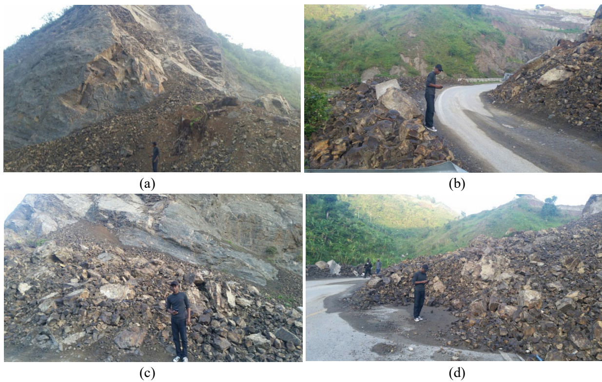
Figure 7.53. Debris flow on RN7 (Lat: 18.4189306, Lon: -73.903528)
