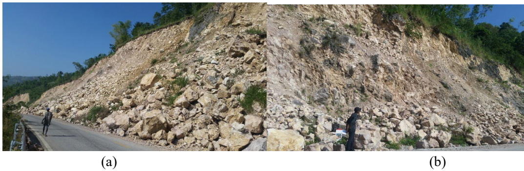
Figure 7.36. Rockfall along RN7 (Lat: 18.374679, Lon: -73.8760854).
