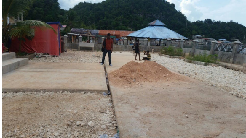
Figure 7.83. Ground cracking near the coast in Pestel (Lat: 18.5422912, Lon: -73.7904188).
