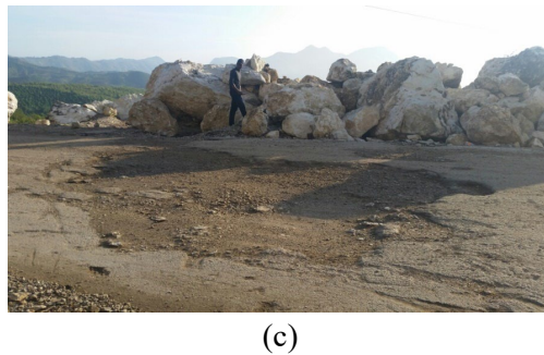
Figure 7.49. Rockfall along RN7 (Lat: 18.4082712, Lon: -73.8832756).
