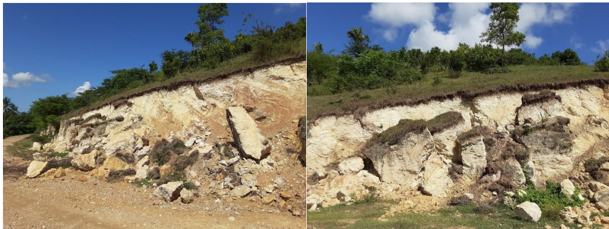
Figure 7.70. Toppling slope failure in Nippes. (a) Lat: 18.43791138, Lon: -73.49213398. (b) Lat: 18.437773, Lon: -73.4922458. Photos taken September 23, 2021.
