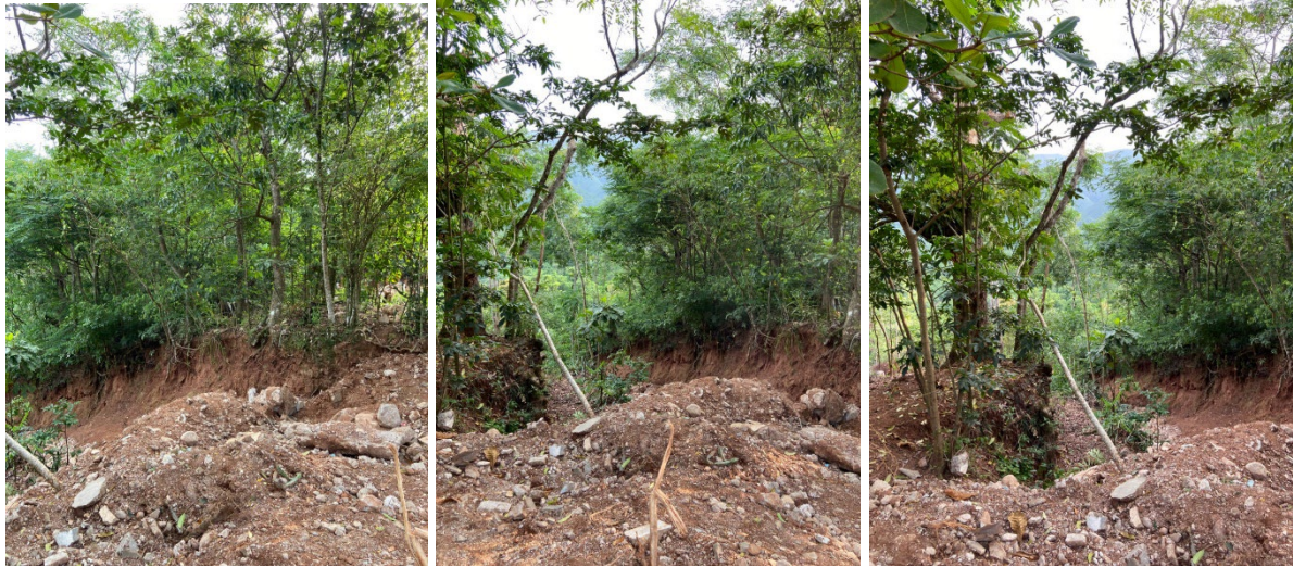
(a) (b) (c) Figure 7.6. Slope failure near Balou (Lat: 18.37866, Lon: -73.51278).
