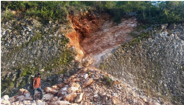
Figure 7.62. Rockslide along RN7 (Lat: 18.4561665, Lon: -73.9199208).
