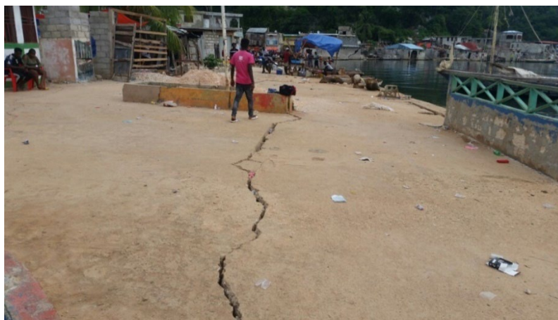
Figure 7.85. Ground cracking near the coast in Pestel (Lat: 18.5424493, Lon: -73.7910169).
