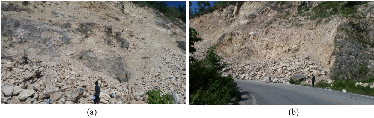
Figure 7.33. Rockfall along RN7 (Lat: 18.3737682, Lon: -73.8769681).
