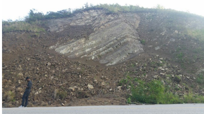
Figure 7.51. Slope failure along RN7 (Lat: 18.4166156, Lon: -73.9020873).
