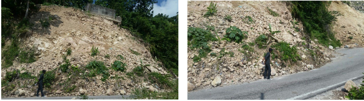
Figure 7.26. Slope failure along RN7 with water tank at top of slope (Lat: 18.3652708, Lon: -73.8791013).
