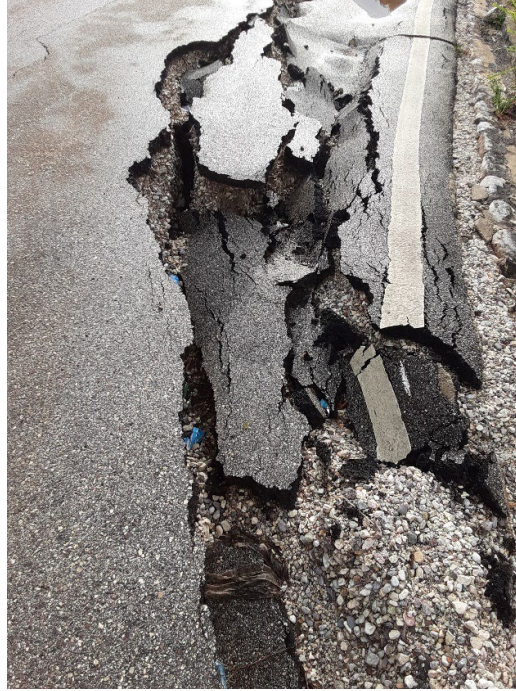
Figure 7.105. Pavement damage on RN7 (Lat: 18.39580833, Lon: -73.87810833). Photo taken September 29, 2021.
