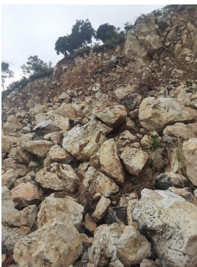
Figure 7.38. Rockfall along RN7 (Lat: 18.376124, Lon: -73.8739723). Photo taken September 28, 2021.
