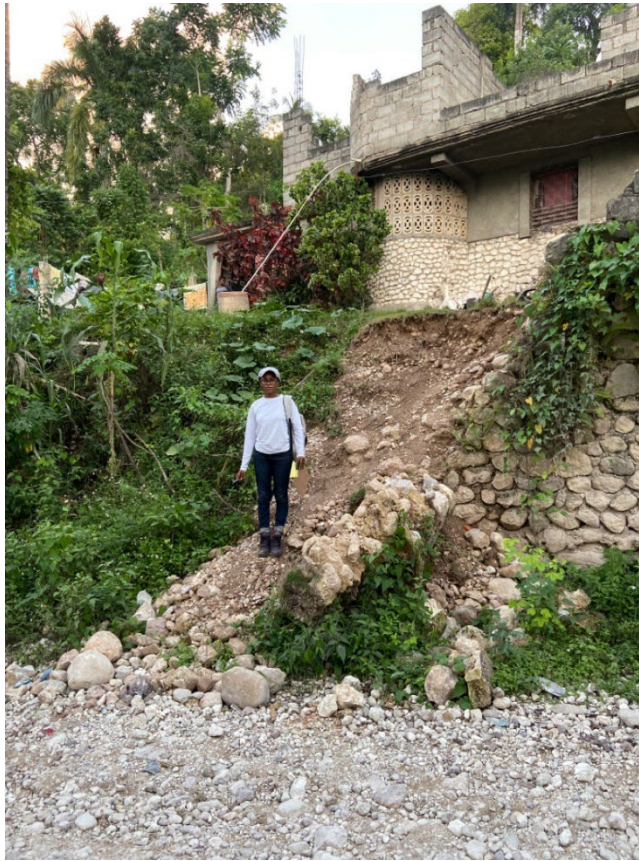
Figure 7.102. Retaining wall damage 2 km north of Enriquillo-Plaintain Garden Fault in Bonne Fin (Lat: 18.38944, Lon: -73.61028).
