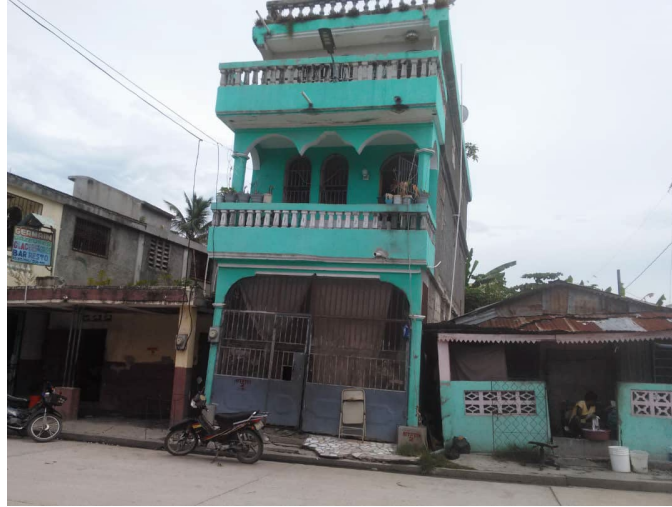
Figure 7.111. Damaged building in Les Cayes (Lat: 18.1944, Lon: -73.7456).
