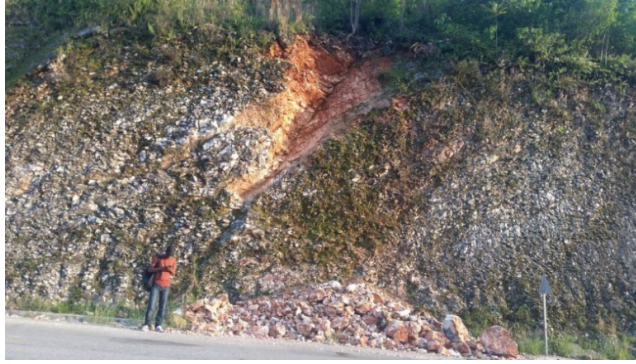
Figure 7.61. Rockslide along RN7 (Lat: 18.456184, Lon: -73.919748).
