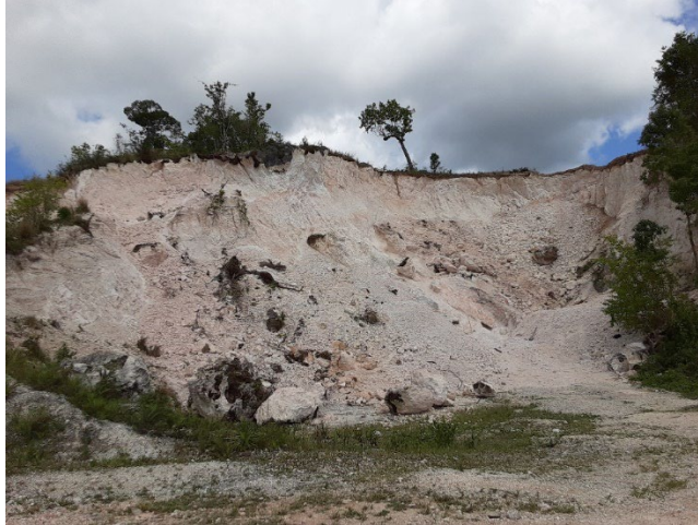
Figure 7.71. Slope failure in Nippes. (Lat: 18.39118189, Lon: -73.54879741). Photo taken September 23, 2021.
