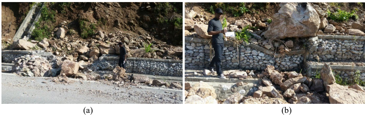
Figure 7.99. Retaining wall damage along RN7 (Lat: 18.403283, Lon: -73.8750032).
