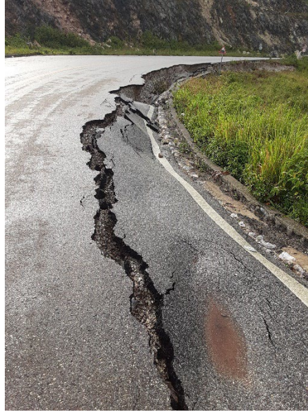
Figure 7.107. Pavement damage on RN7 (Lat: 18.40532455, Lon: -73.87818961). Photo taken September 29, 2021.
