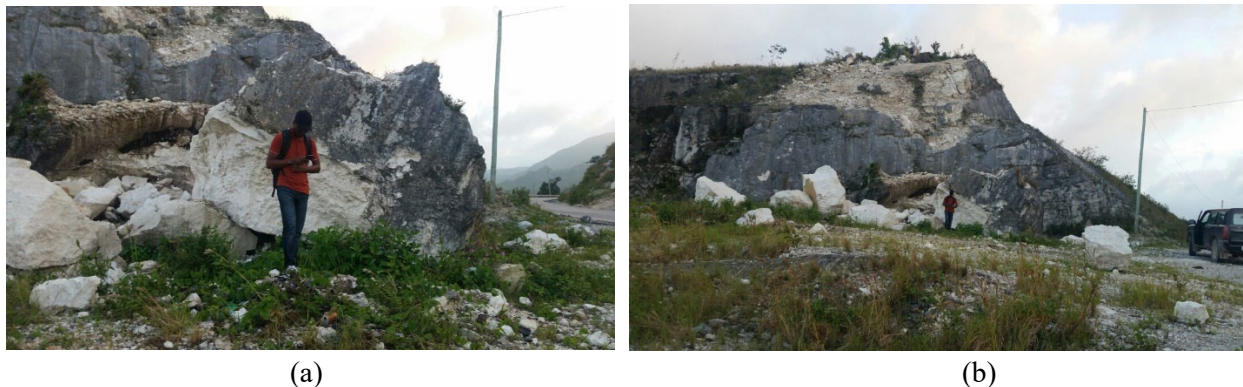
Figure 7.58. Possible failure of rockface along RN7 (Lat: 18.429466, Lon: -73.8998361).
