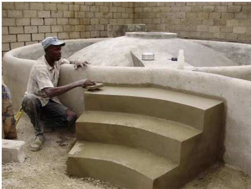
Figure 6 biodigester à Kaynou, Belair
