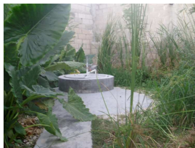
Biogas Unit or Biodigester
