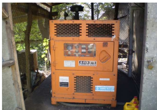
Biogas powered generator
